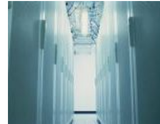
Media, Communications iDC
